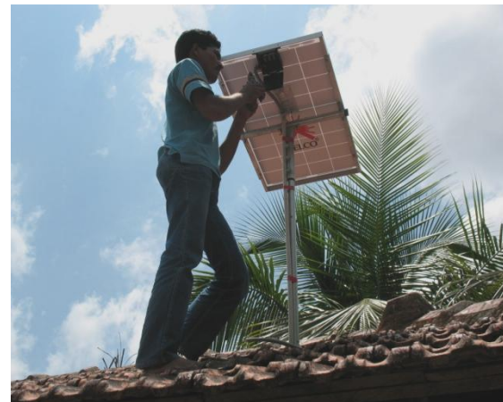
A typical Solar Home Lighting System installation by SELCO in a rural town near Kundapur, Udipi District
